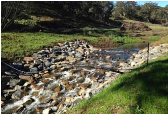
Fig 1: Grade stabilisation structure (rock ramp) with protective grass cover establishing around it.
