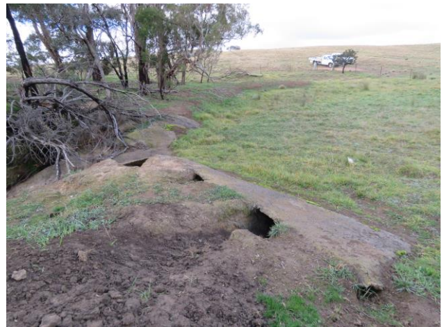
Fig 2: Burrowing under a flume apron may cause it to fail
