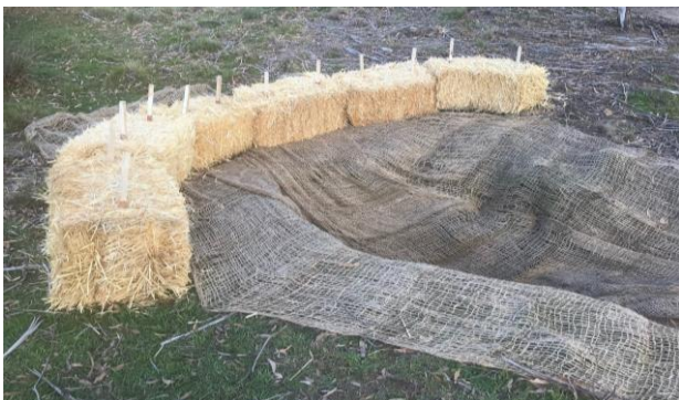
Fig 1: Jute mesh installed with hay bales to divert water away from an active erosion point.
