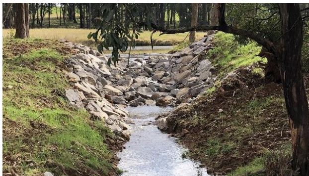
Fig 3: Rock ramp guides flow safely to centre of gully.
