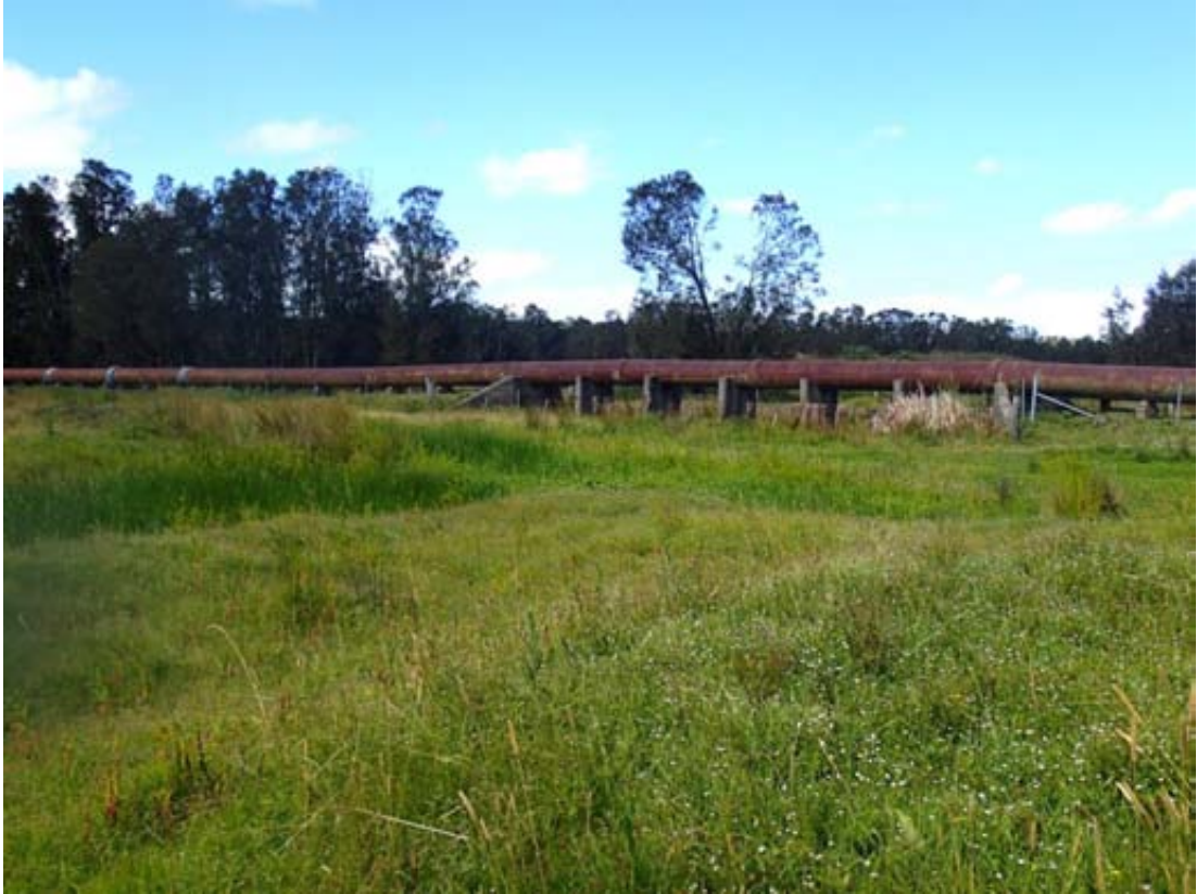
Figure D.11: P10 – HWC pipeline
