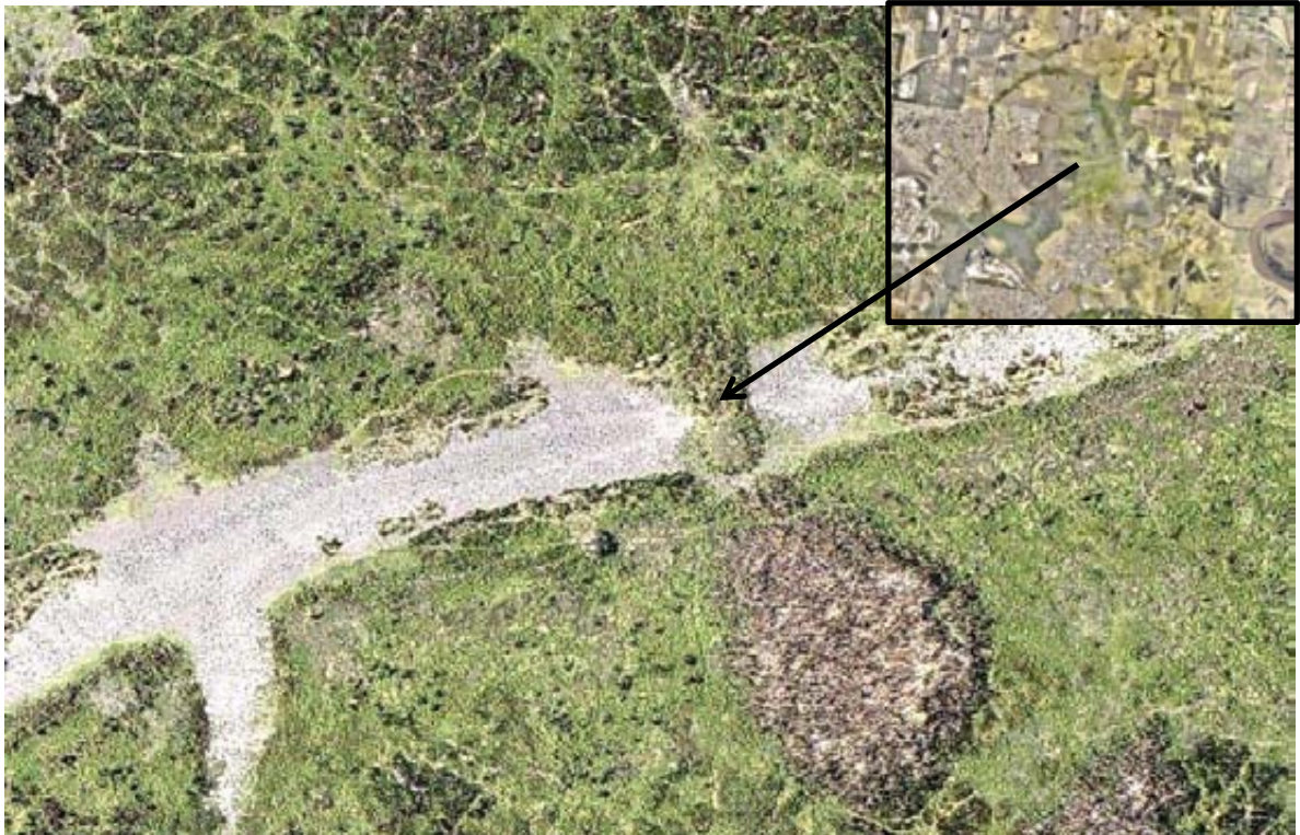
Figure 3.5: Collapsed culvert in the middle of the floodplain (Background image: Near Map)
