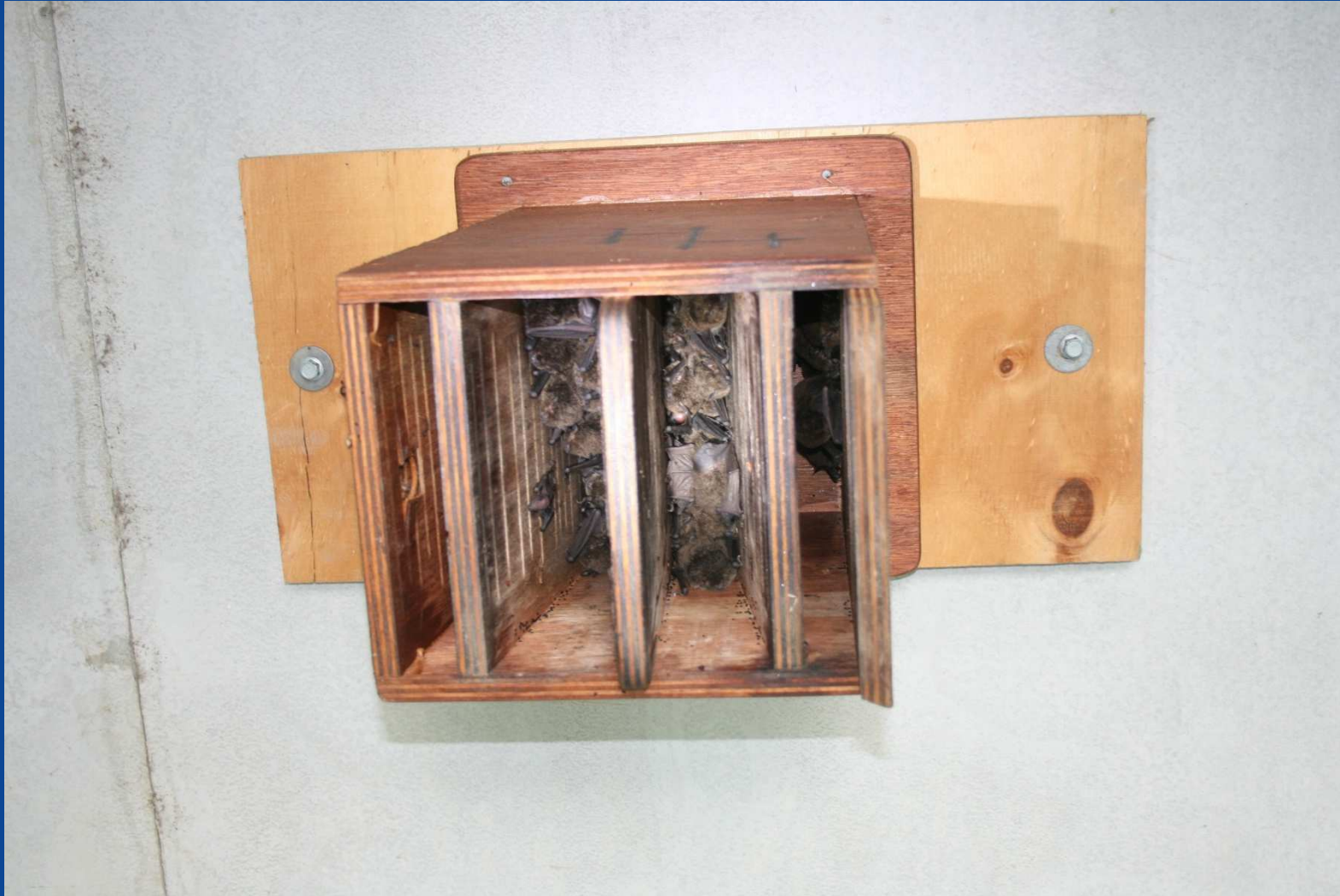
Multi-chambered bat box Installed in culvert. Photo: Veronica Silver.
