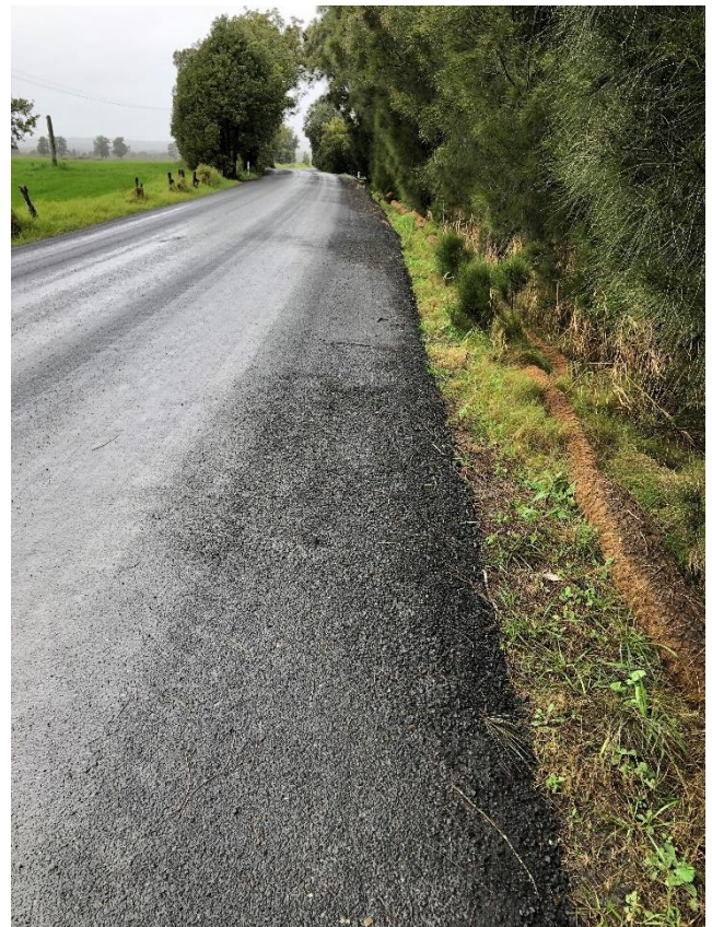
Figure 2. Mayfield Road after works to seal it were completed, with sediment no longer running into nearby waterways.
