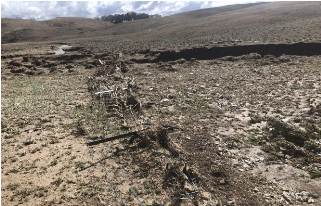
Figure 4: Increased run-off in this fireground has trapped debris in a hinge joint fence, now needing to be replaced.
