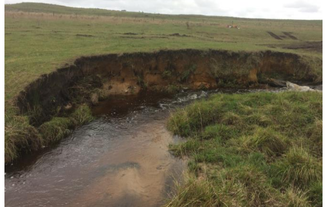
Figure 5: Low groundcover higher in the landscape leading to powerful waterflow has scoured the base of this creek bank on a tight bend. This can be difficult to control, and approvals may be required, so seek LLS advice.
